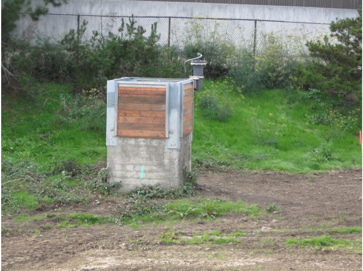
Figure 4: View of overflow weir box structure and water level sensor, showing welds on the steel structure that increased the elevation and capacity of the equalization ponds.
