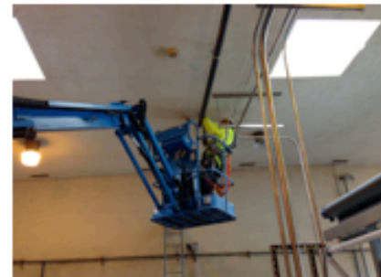
The New Belt Filter Press in Operation
